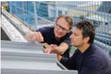
Zambelli RIB- ROOF_Akustikdach_05
