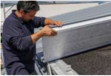
Zambelli RIB- ROOF_Akustikdach_04
